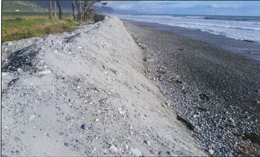
Looking south along the reconstructed Mokihinui SRA sacrificial seawall. The neighbouring landowner Sos Morgan's seawall starts at the pine trees.
